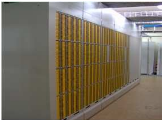
Central Office placement of NeXa
