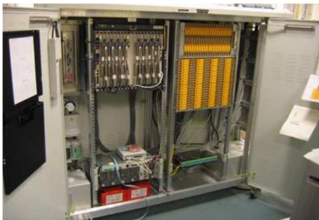
Street Cabinet placement of NeXa
