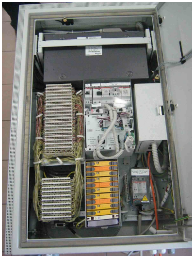
In-building placement of NeXa
